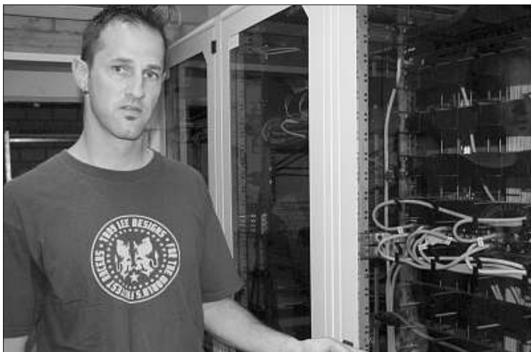
Passa 10 kilometers cabels han ins duvrà sco ch'il specialist Hanspeter Gujan mussa per tut ils novs indrizs electronics.
